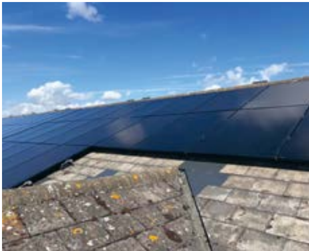
Solar panels on the Russell Street roof
